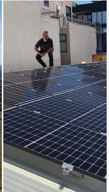
The Rubato Building's 15kW solar panels have been installed with assistance from Council.
