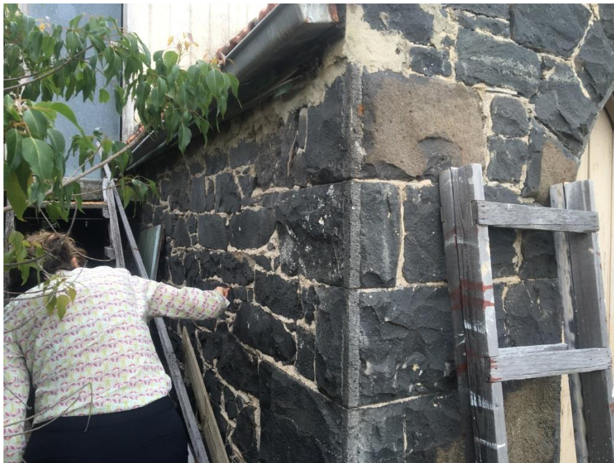
Figure 15: Bluestone coursing is consistent with nineteenth-century building materials and techniques (source: Context 2016)
