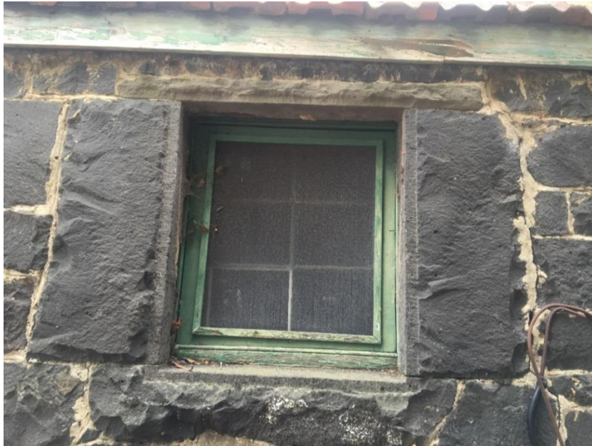
Figure 14: Victorian window flanked by large bluestone blocks and topped with sandstone (source: Context 2016)
