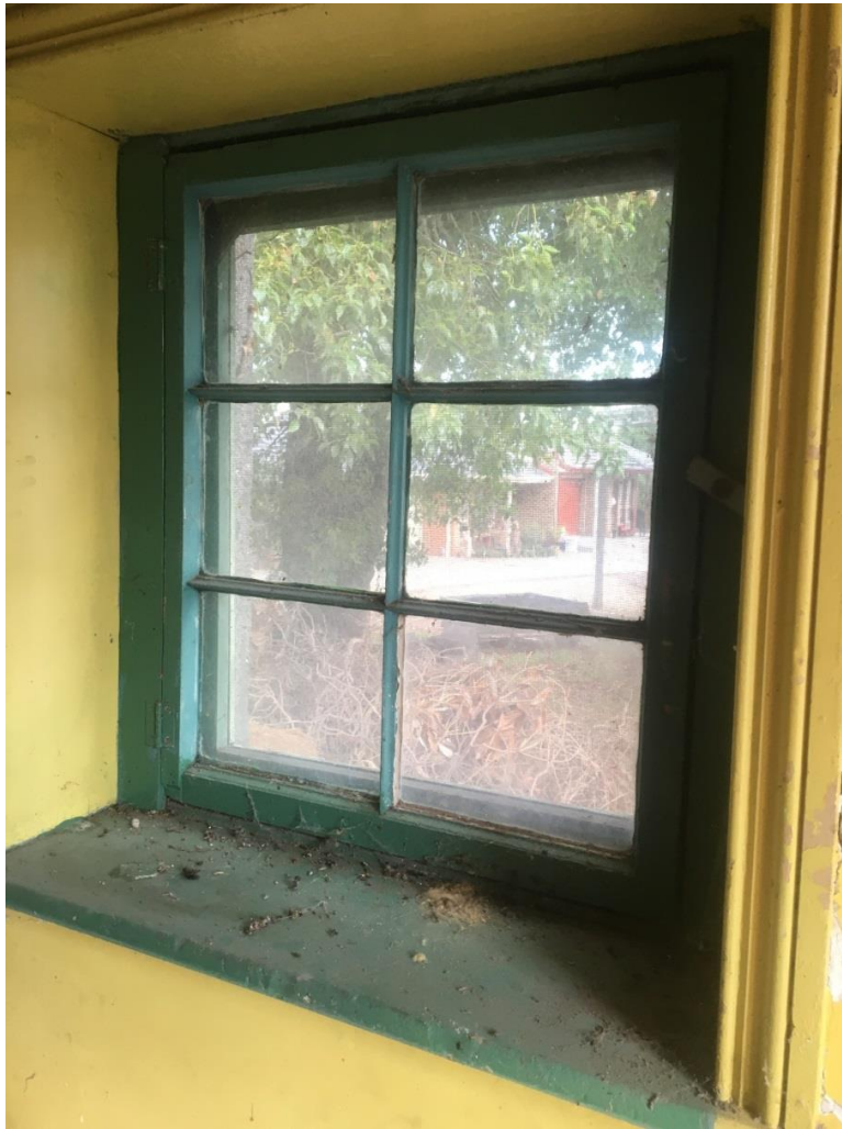
Figure 18: Victorian-style window with 'lamb's tongue' profile glazing bars on the south side of the outbuilding (source: Context 2016)
