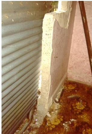
Photograph of Monolithic reinforced concrete wall with flared base, 36 King Street, North Fitzroy (source: Paul Roser, 'Concrete Houses')
