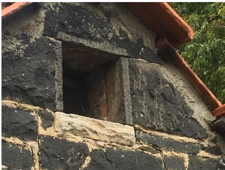
Figure 17: There is evidence of bricks in the lining of the building (source: Context 2016)
