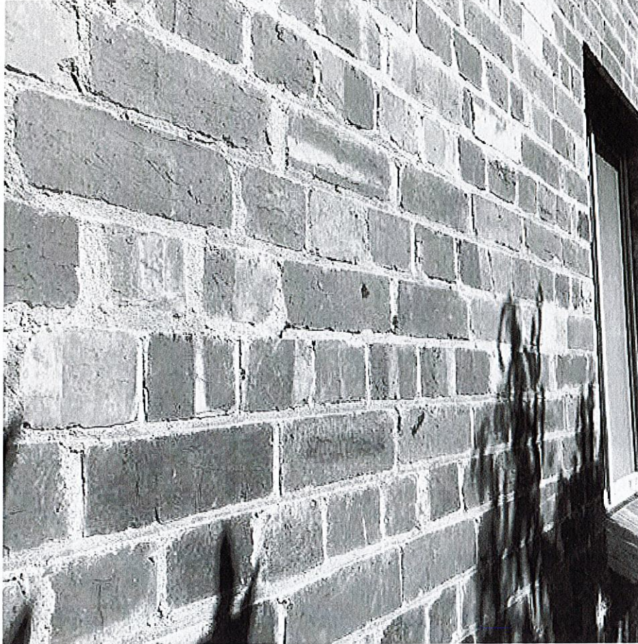
Middle portion of the east elevation rebuilt in an English brick bond.
