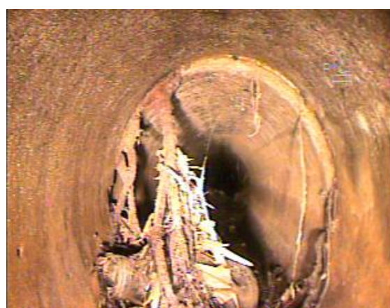
Photo 2 – Tree roots entering Council's underground pipe via cracks or at butt joints and causing blockages and displacement of the pipe.
