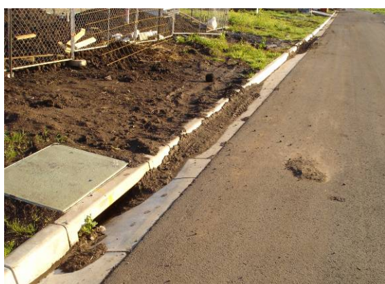
Photo 3 – Debris from building sites entering the underground drainage system.
