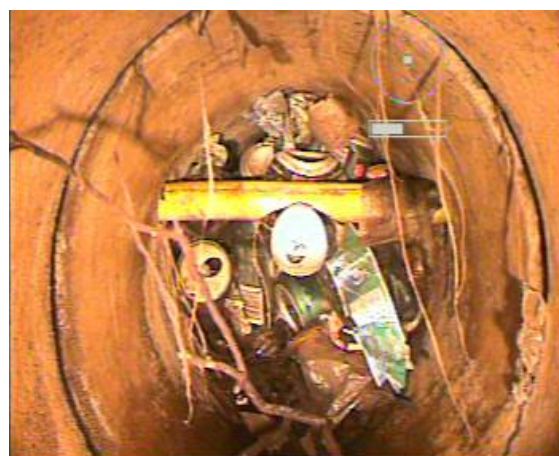
Photo 1 – Service authority conduit passing through Council's underground pipe and causing blockages.
